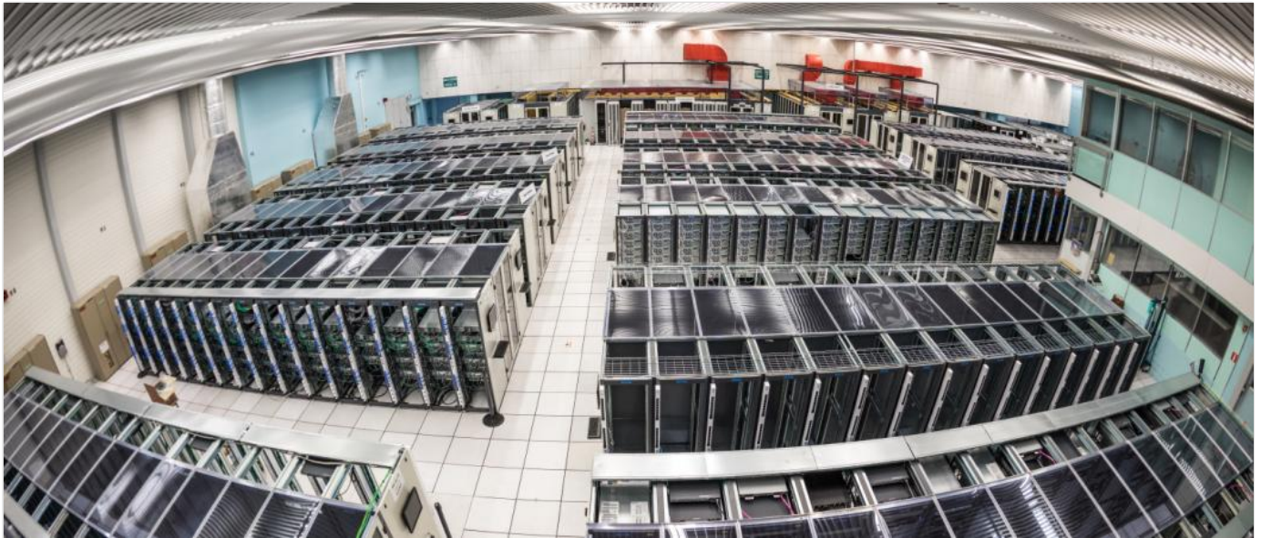
CERN Data Centre. Photo: CERN
